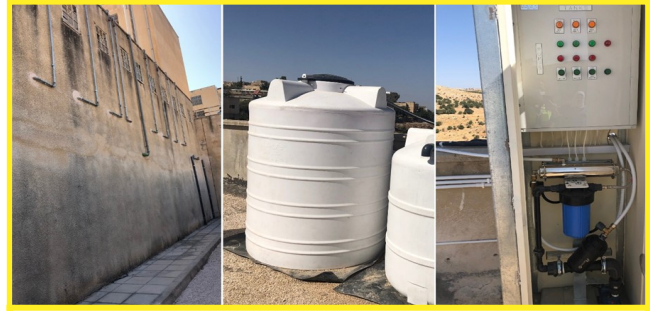
The greywater treatment system at Samir Al-Rifai School
