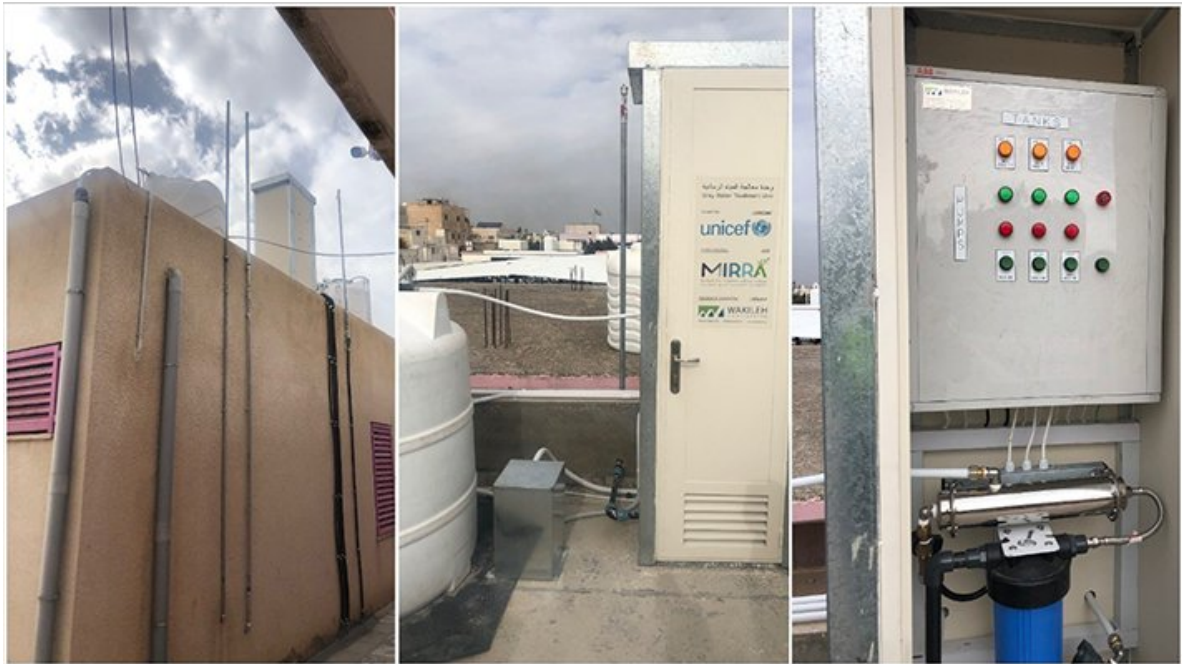
The greywater treatment system installed on the roof of one of the beneficiary schools.
