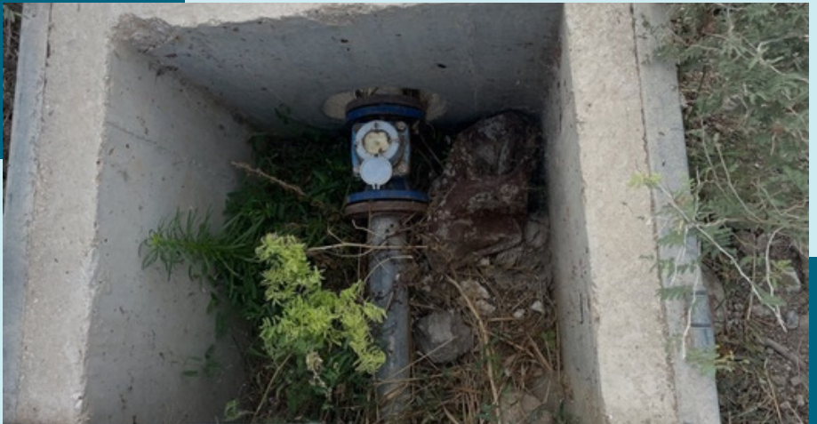
Picture 3: A Farm Turnout Assembly (FTA), which includes a meter and flow limiter and is contained within a concrete box.
