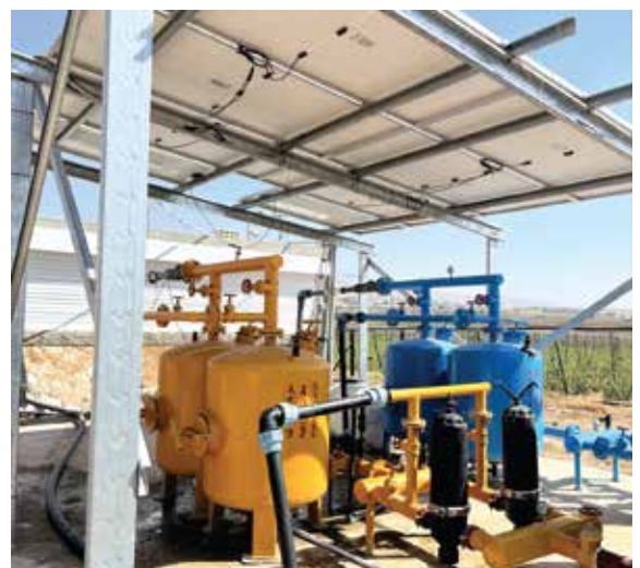
An Automated Solar Water Pump at MIRRA's Climate-Smart Farm
