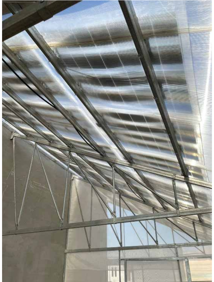
Semi-Transparent Solar Panels from AZMUD Partner, SmartWall in France installed at MIRRA's Climate-smart Farm in the Jordan Valley
